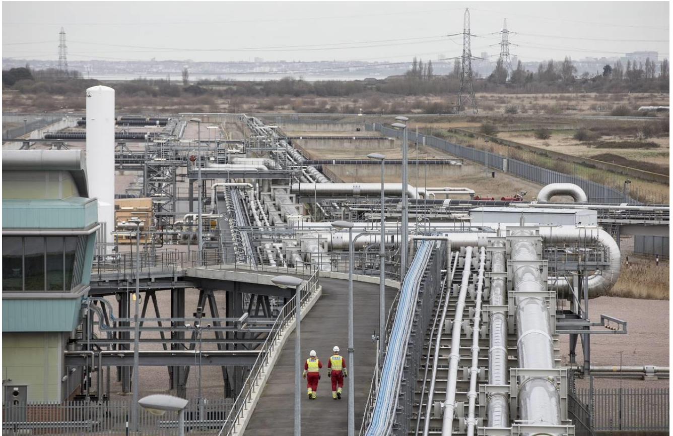
Natural-gas futures have fallen sharply this year, reversing one of last year's most profitable trades. Above, a natural-gas pipeline in the U.K. Photo: Bloomberg News
